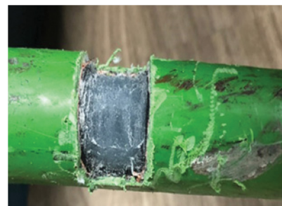
Fig. 9. (Color online) A cable defect with a central angle of 180°, penetration depth of 50% and length of 2 cm; (a) Defect modeling, (b) Photograph.
