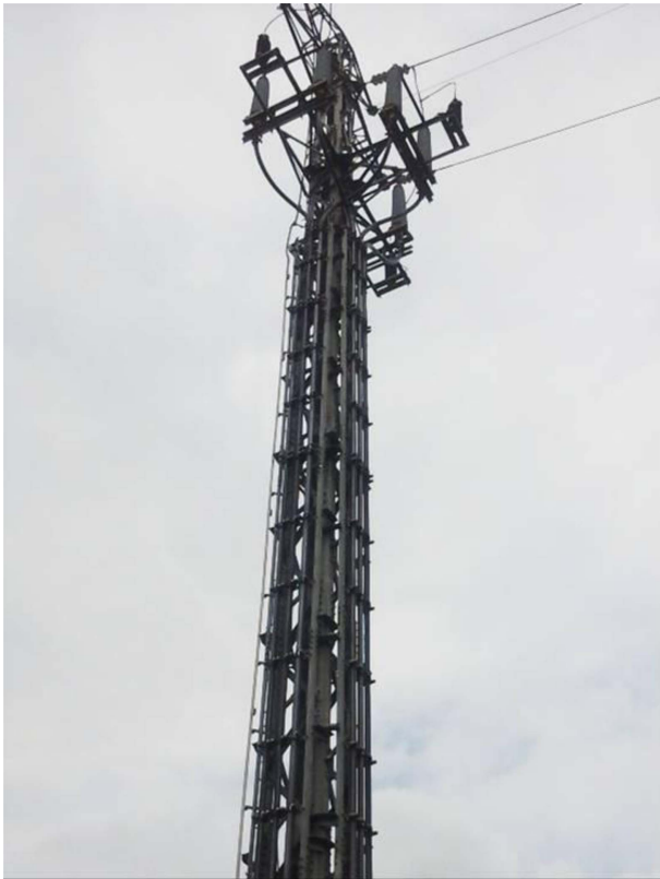
Fig. 2. (Color online) Junction tower with structural steels and cables.
