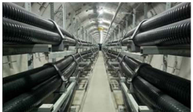
Fig. 1. (Color online) Underground transmission lines.
